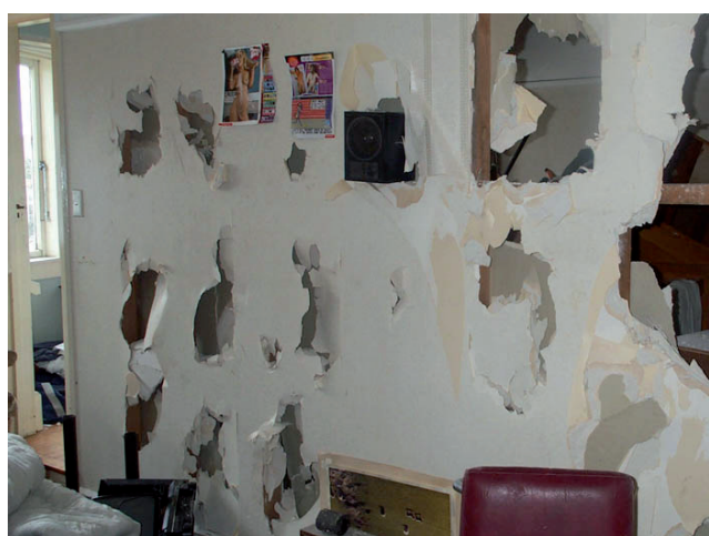
Damaged HNZN flat
